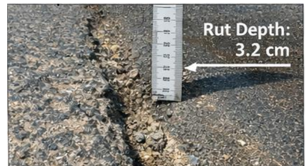
Figure 2. Rut depth measurement on the road surface.
